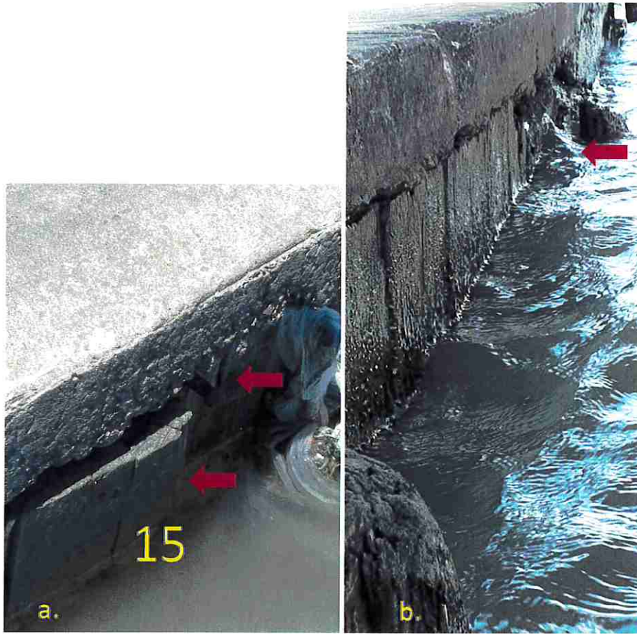
Figure 3: Signs of Decay and Bowing in Existing Timber Bulkhead
